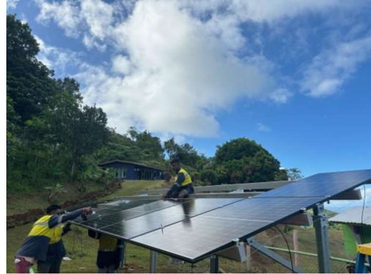
Rabi Island solar project, Fiji
